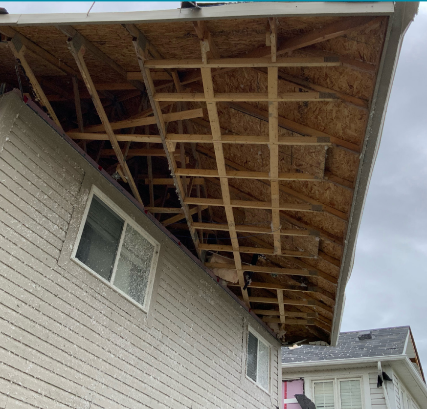
Barrie, ON, 2021 EF2 Tornado Event. Credit: GA Kopp, UWO.
