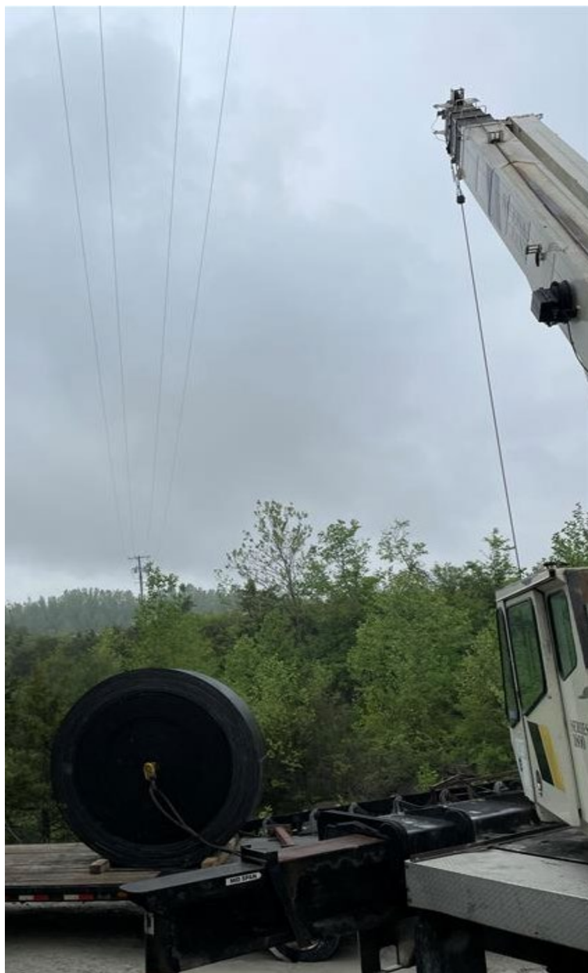
APPENDIX C – Photo of Roll of Belt Positioned under High-Voltage Powerlines
