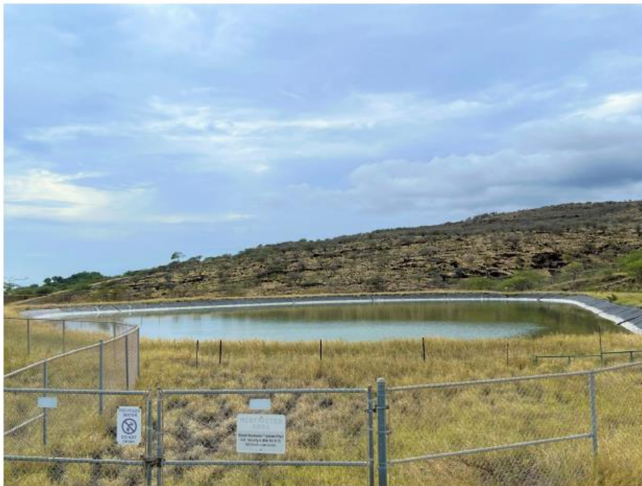
Open pond at the Mānele Wastewater Treatment Facility
