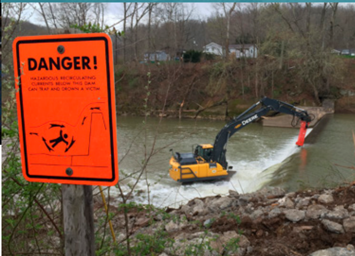
(Top) Removal of the Highland Dam on the West Fork River in West Virginia.
