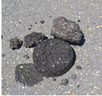
Figure 75. Photo. Asphalt concrete layer cores taken from wheel path; I-25, Colfax County, New Mexico.
