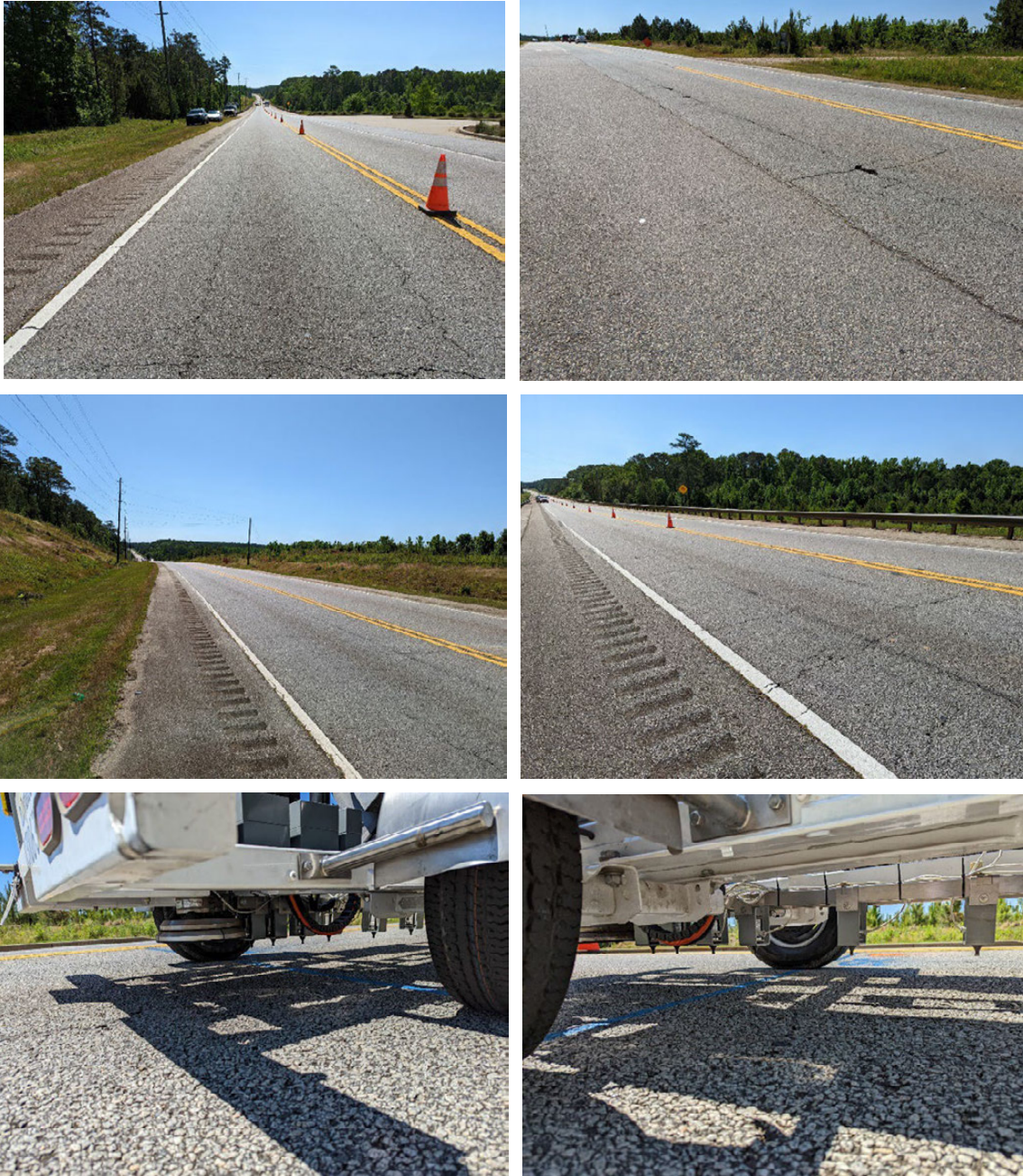
Figure 129. Photo. Inverted pavement westbound lane also showing FWD test setup in May 2022; LaGrange Bypass Road, Georgia.
