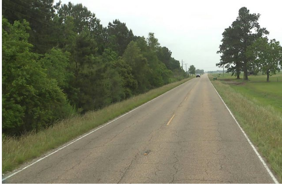
Figure 14. Photo. Reflective shrinkage cracks in the form of block cracking on LA-97 (LaDOTD).
