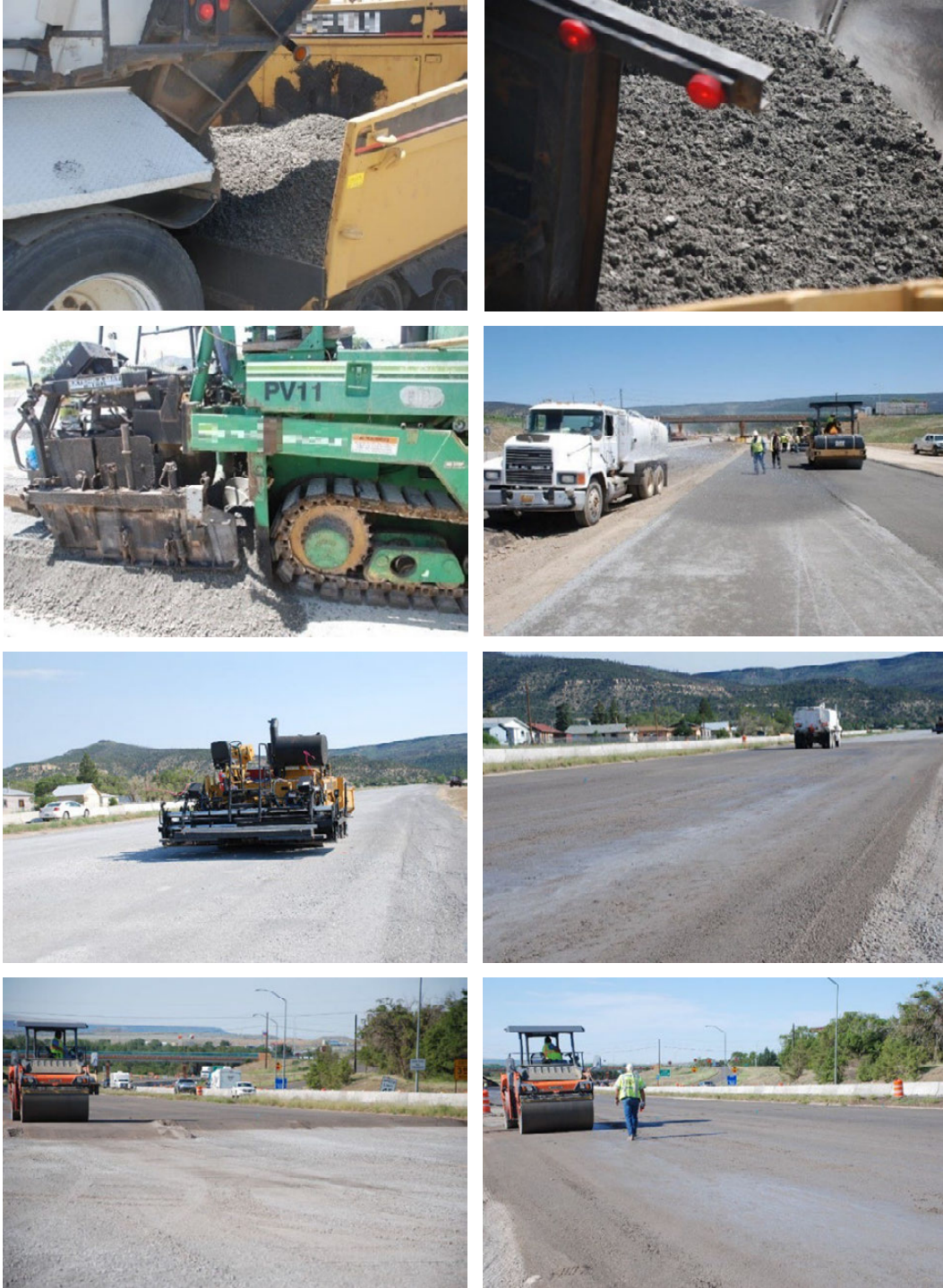
Figure 23. Photo. Cement-treated base construction; I-25, Colfax County, New Mexico (credit: Bryce Simons).
