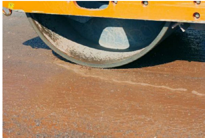
A. Excess fines being expelled as slush from layer.
