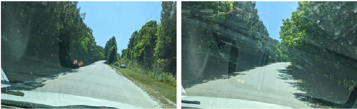
Figure 140. Photo. South African inverted pavement in the outbound lane in May 2022; Morgan County Quarry Access Road, Georgia.
