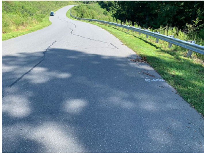
B. Longitudinal crack (IP, Station 5+50).
