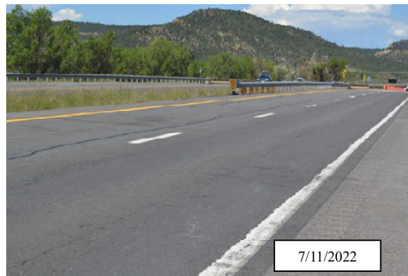
Figure 70. Photo. Part of the northbound section left with the blade patch; I-25, Colfax County, New Mexico.
