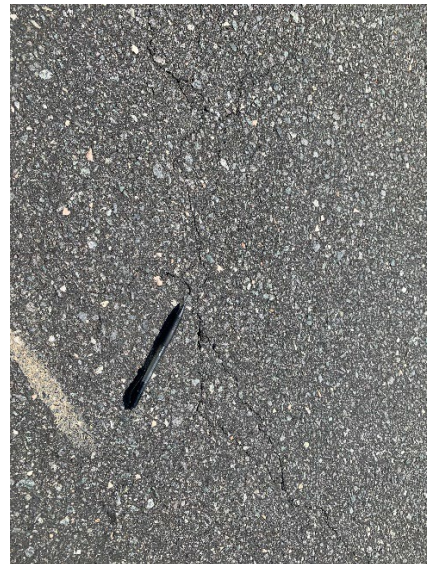
D. Fatigue cracking (CP, Station 14+50).
