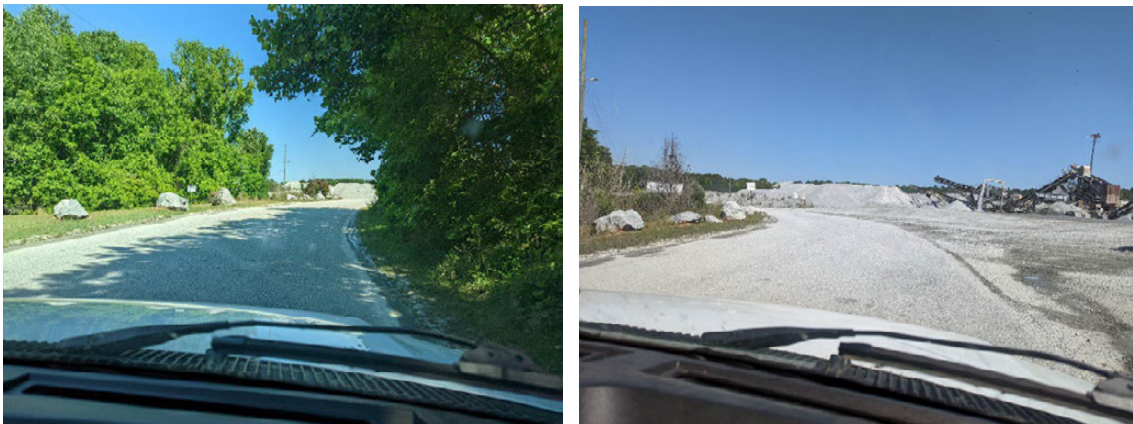
Figure 141. Photo. Georgia inverted pavement in the inbound lane in May 2022; Morgan County Quarry Access Road, Georgia.
