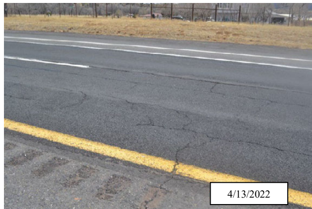
Figure 68. Photo. Transverse and longitudinal cracks connecting to form block cracking pattern; I-25, Colfax County, New Mexico.
