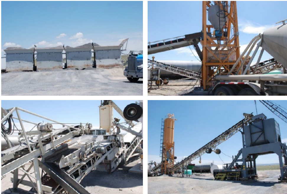
Figure 26. Photo. Granular base course batch plant for I-25, Colfax County, New Mexico (credit: Bryce Simons).
