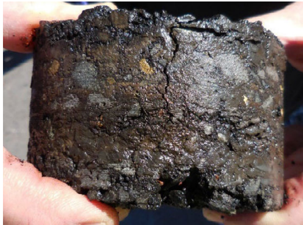
E. AC core showing top-down cracking.
