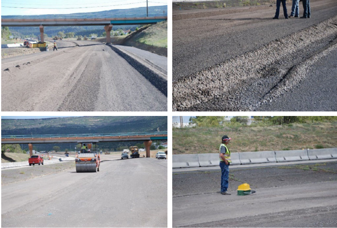
Figure 28. Photo. Granular base course construction at I-25, Colfax County, New Mexico (credit: Bryce Simons).
