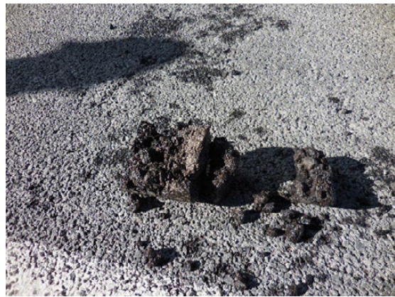
D. Pavement core showing AC stripping.
