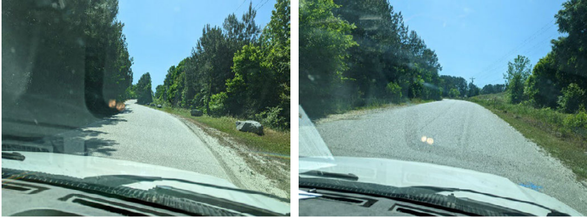
Figure 142. Photo. Georgia inverted pavement in the outbound lane in May 2022; Morgan County Quarry Access Road, Georgia.
