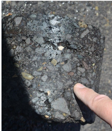
Figure 74. Photo. Bottom-up cracking observed in a field core obtained from northbound lane; I-25, Colfax County, New Mexico.
