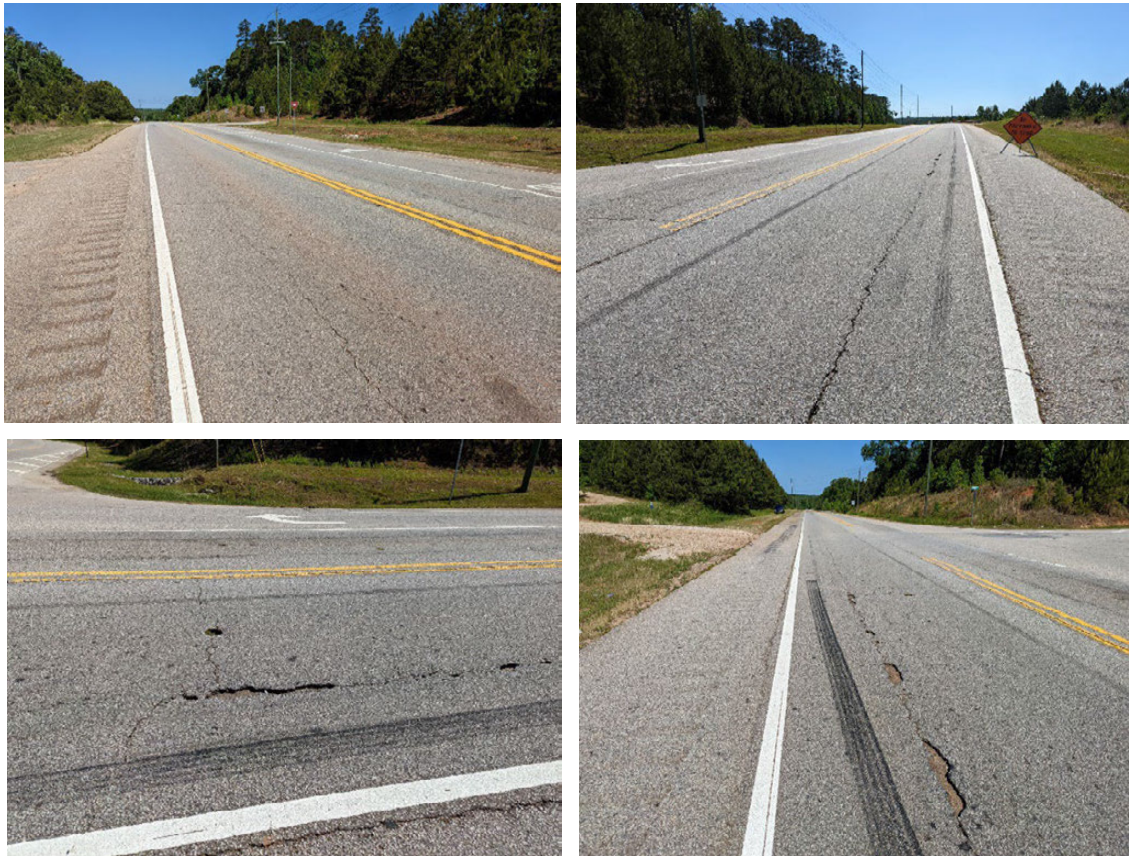
Figure 128. Photo. Inverted pavement eastbound lane in May 2022; LaGrange Bypass Road, Georgia.
