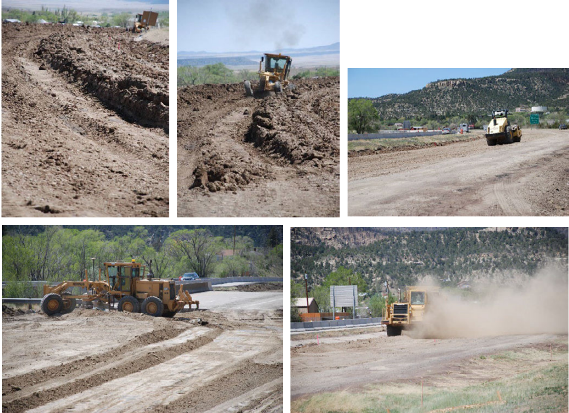
Figure 22. Photo. Subgrade preparation at I-25, Colfax County, New Mexico (credit: Bryce Simons).
