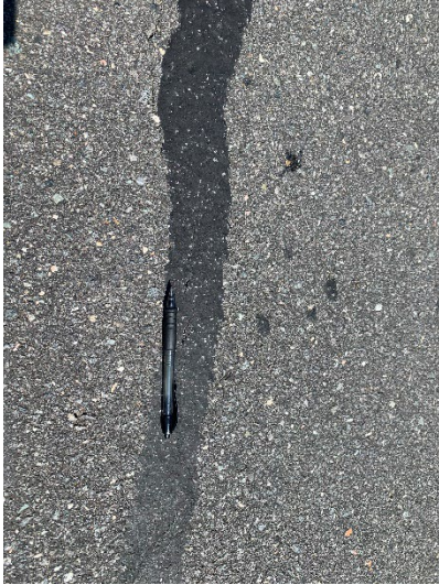
A. Transverse crack (IP, Station 4+91).
