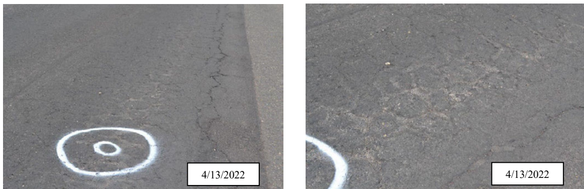
Figure 65. Photo. Northbound inverted pavement section patched lane showing reflecting wheel path fatigue cracks; I-25, Colfax County, New Mexico.
