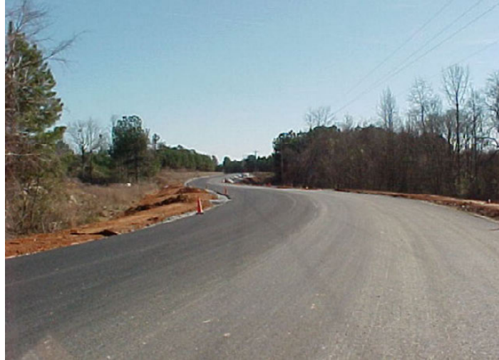
Figure 135. Photo. Inverted pavement section constructed in Morgan County, Georgia, in 2001 (TRB Webinar 2016).
