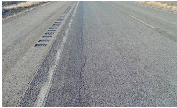
B. Longitudinal cracking within wheel path.
