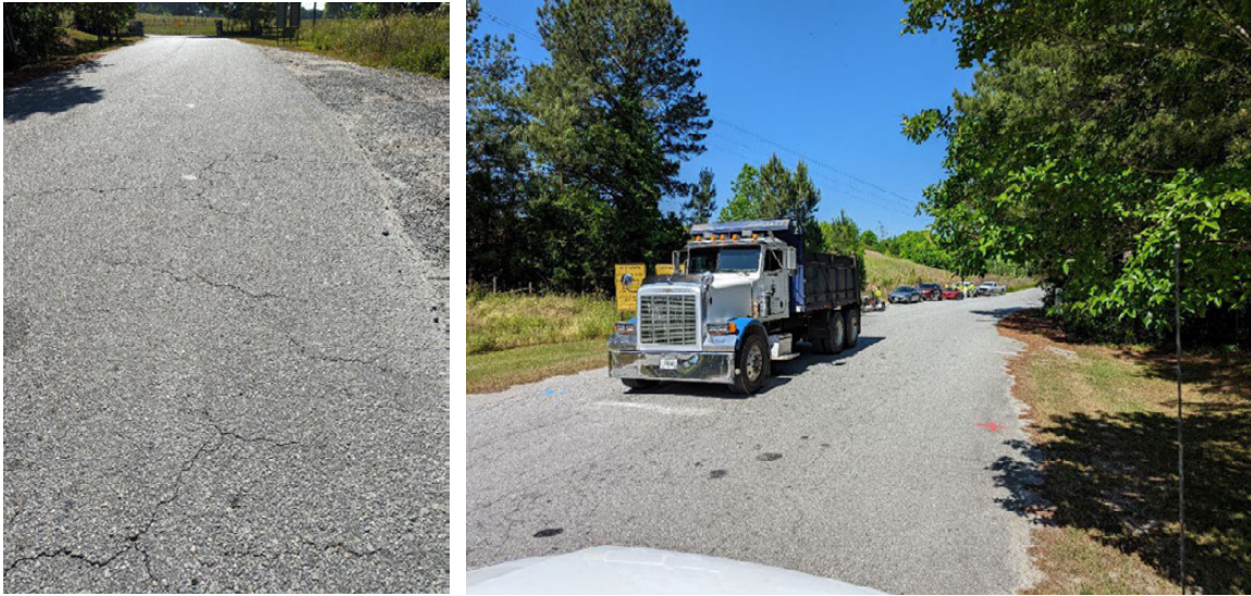
Figure 137. Photo. Conventional pavement in the inbound lane in May 2022; Morgan County Quarry Access Road, Georgia.
