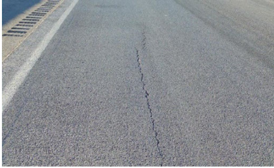
A. Longitudinal cracking outside wheel path.
