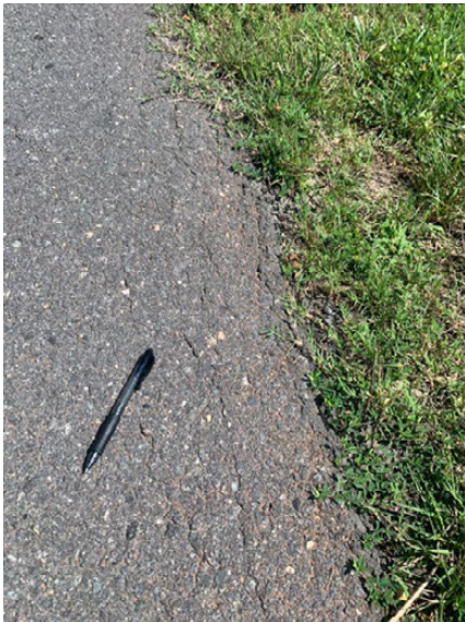
C. Edge cracking/deterioration (CP, Station 10+00).
