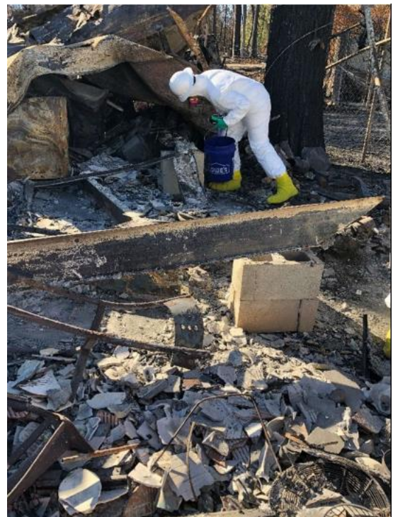
Environmental Protection Agency contractor investigates hazardous materials on property damaged by Oregon wildfires.
