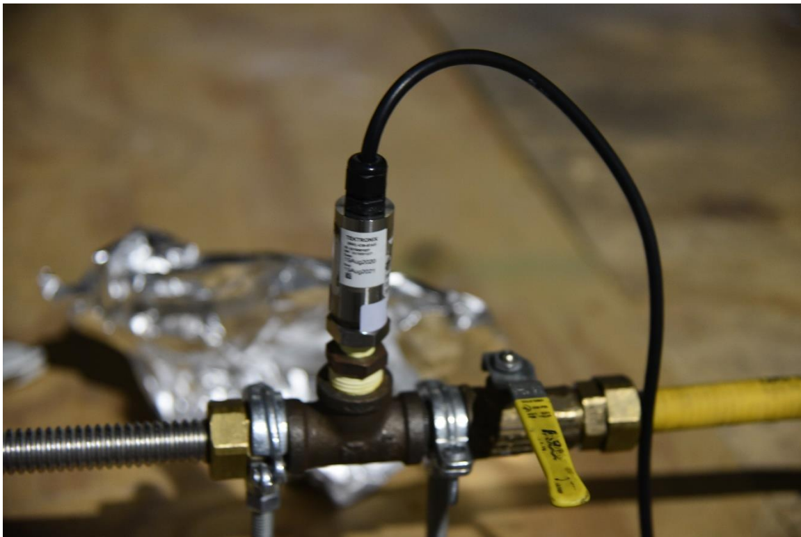
Figure 10. Pressure transducers (348035_1191810.jpg)
