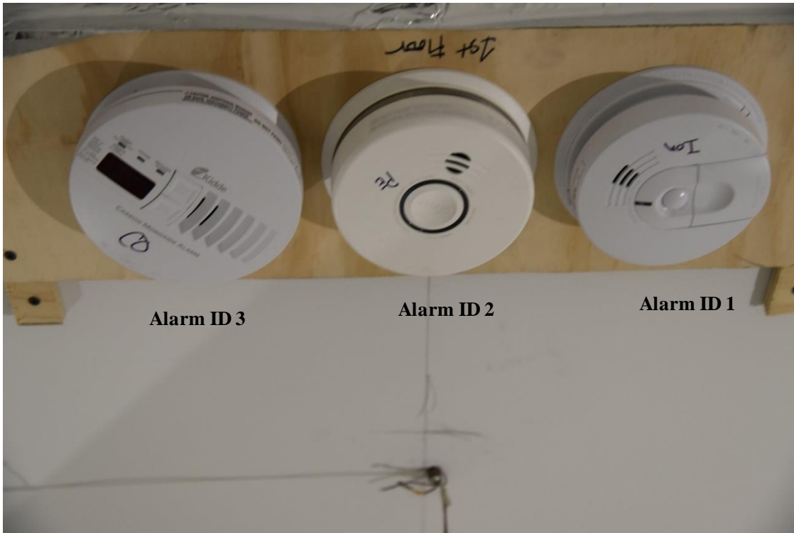
Figure 16. AC powered alarms – image annotated (360079_1304666.jpg)
