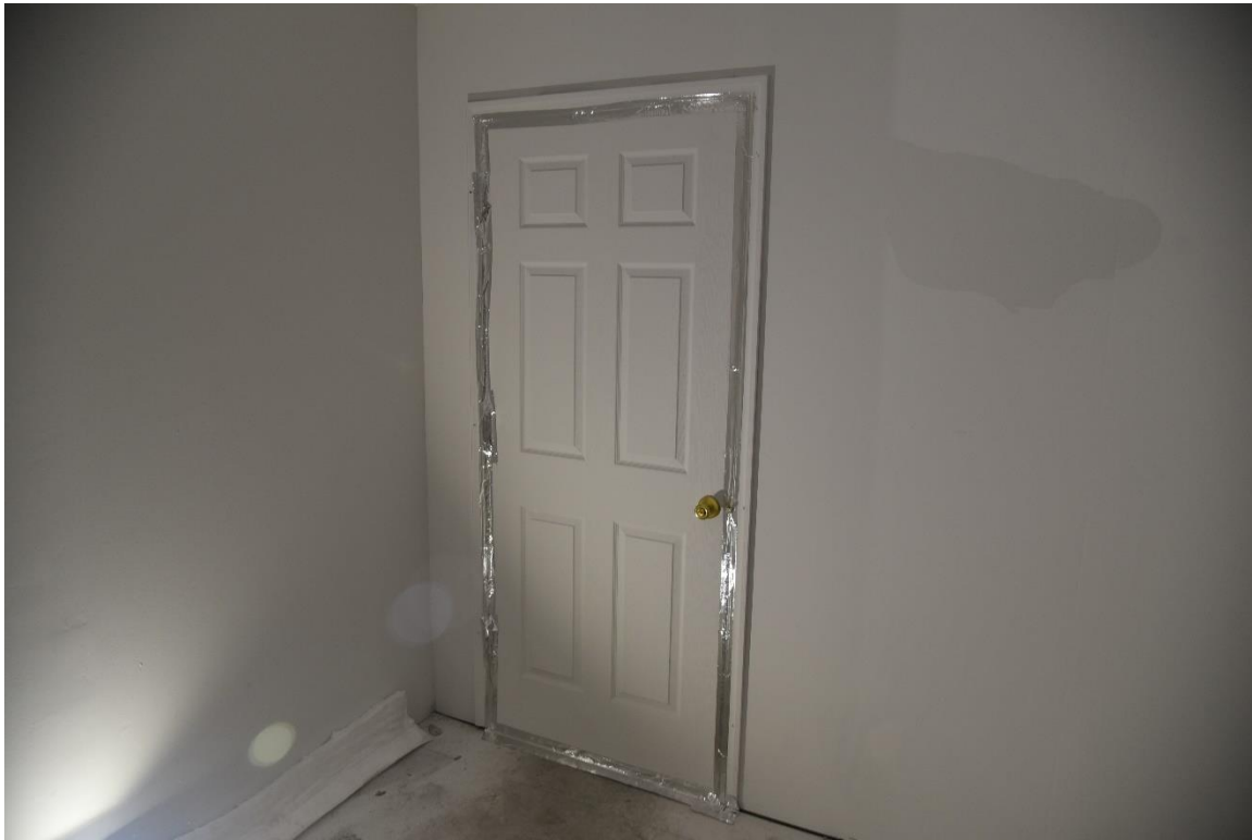
Figure 5. First floor door sealed with aluminum tape (360079_1304764.jpg)
