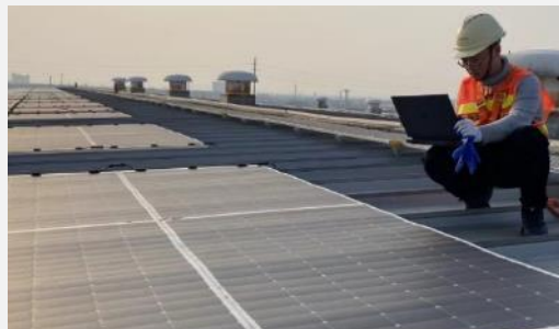
Rooftop solar panels at Mapletree Wuxi New District Logistics Park, China
