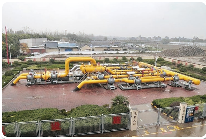
Smart Gas Station – Hangzhou Hezhuang Gas Supply Station* (河莊供氣站)
