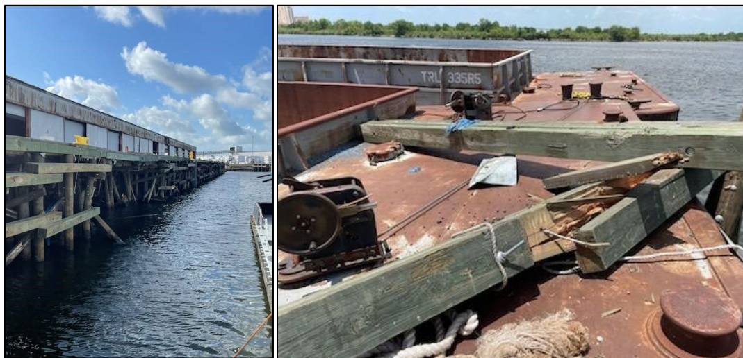
Figure 4. Left to right: Damage to the Port of Lake Charles pier, and timber from the pier found on the starboard lead barge of the Danny Terral . (Source: Coast Guard)
