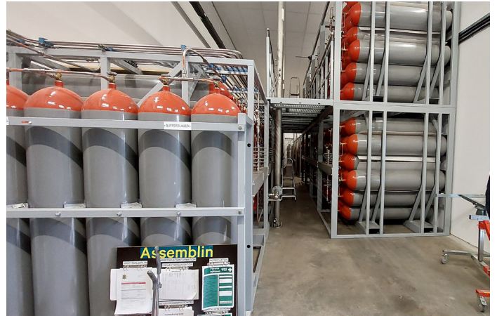
Gas buffer storage at the bus depot in Uppsala. Photo: OST
