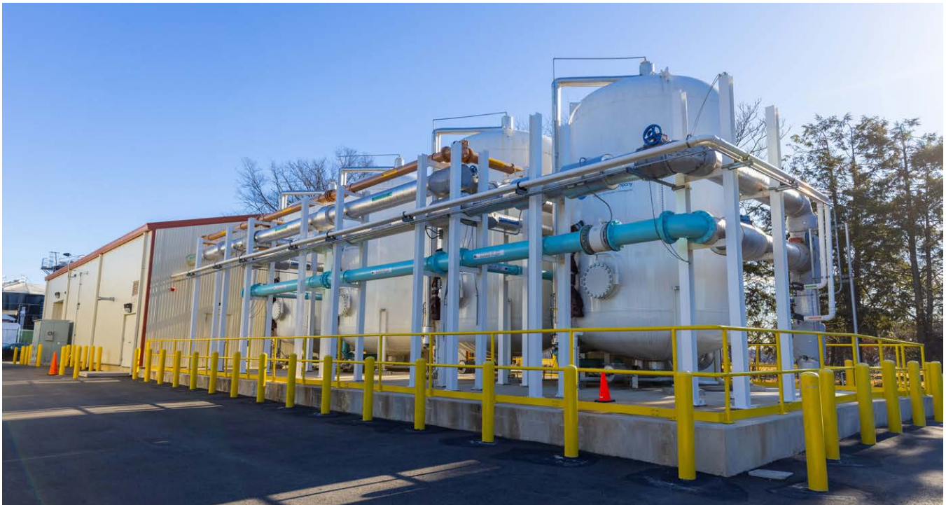
PFAS treatment at American Water facility in Camden, NJ
