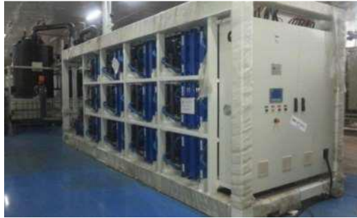
400 MWh VRFB from Pu Neng in Hubei
