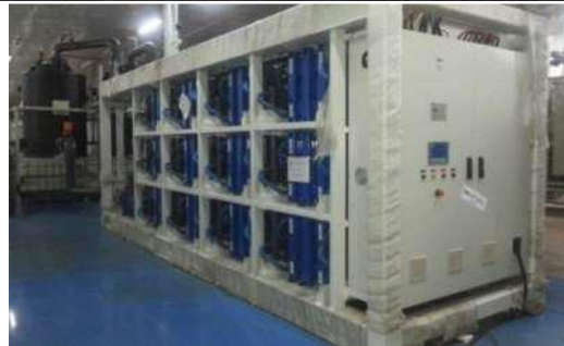
400 MWh VRFB from Pu Neng in Hubei
