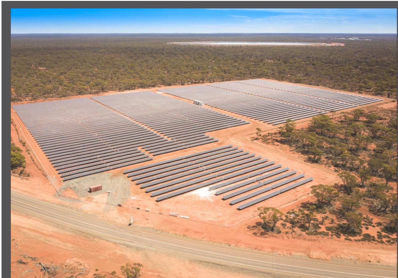
Zenith currently constructing 2MW solar energy and battery farm at KOTH (similar Zenith power installation shown in picture)
