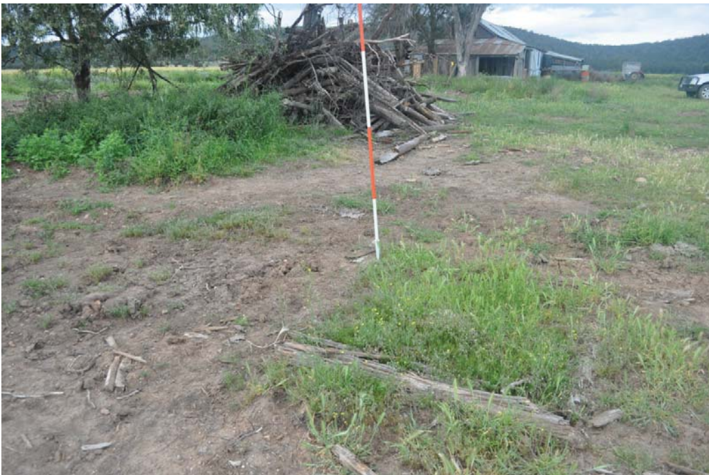
Figure 33: Remains of the plunge sheep dip. Demolition of structures adjacent to the Velyama Shearing Shed has occurred recently and remains piled up or pushed into a waterway at the rear of the shed.
