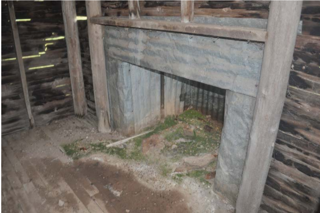
Figure 55: Fireplace constructed of round logs and galvanised iron – Warriahdool hut, October 2010.
