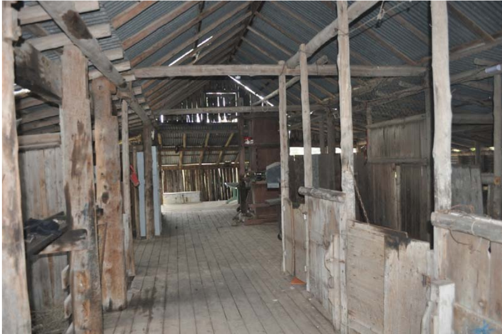
Figure 23: The Velyama Shearing Shed is substantially intact. Parts of the shearing plant, wool classing tables and other mechanical items have been removed to outside the shed.
