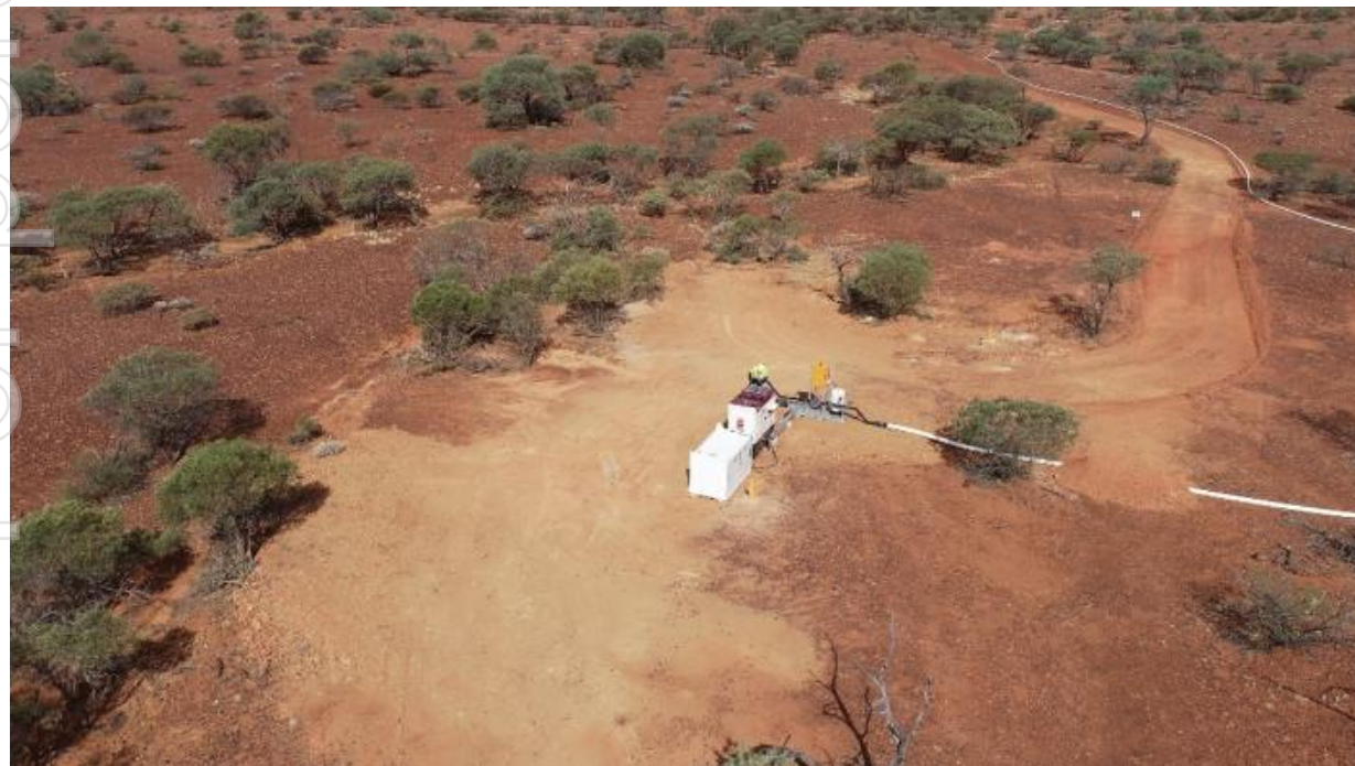
SipHon Borefield - Fully permitted consisting of 6 bores, fully equipped with holding tanks and high flow pumps and pipeline to the process plant.
