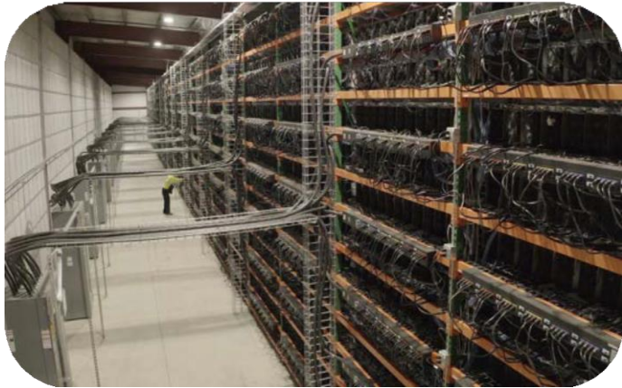
Jamestown, North Dakota Facility 106MWs
