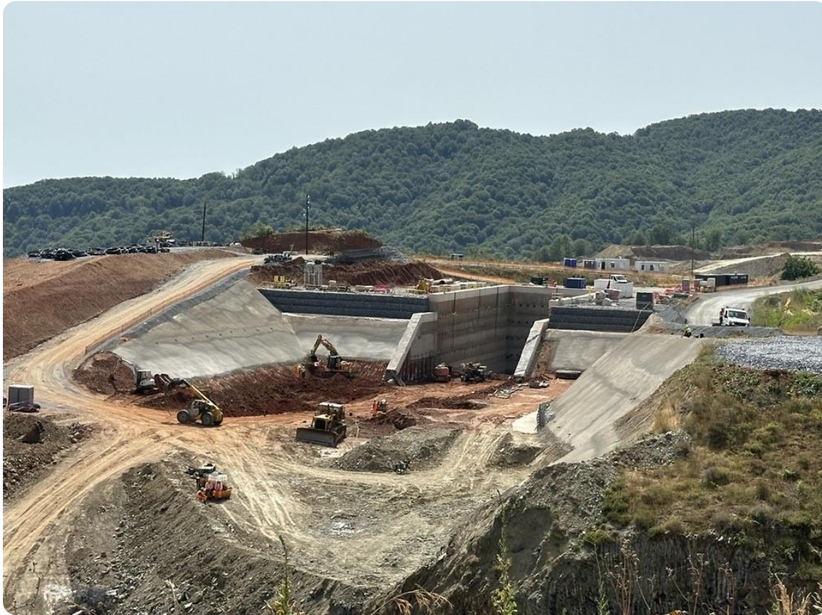
Excavations and slope stabilizations are progressing in all areas and the excavation and backfill for the conveyor alignment is in progress (not shown on the above image).
