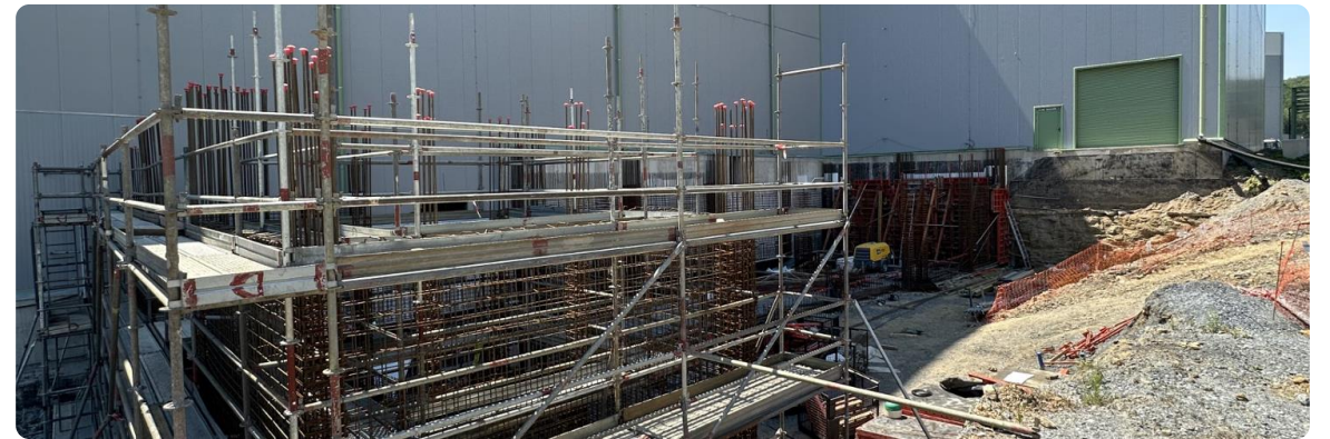
Process Control Room
