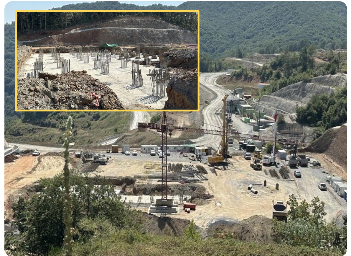
Two active drills are working at the filter plant, where 270 piles have been completed. The inset photo shows a closer view of the piles. A 3 rd drill has recently arrived on site and it is currently undergoing inspection ahead of use.
