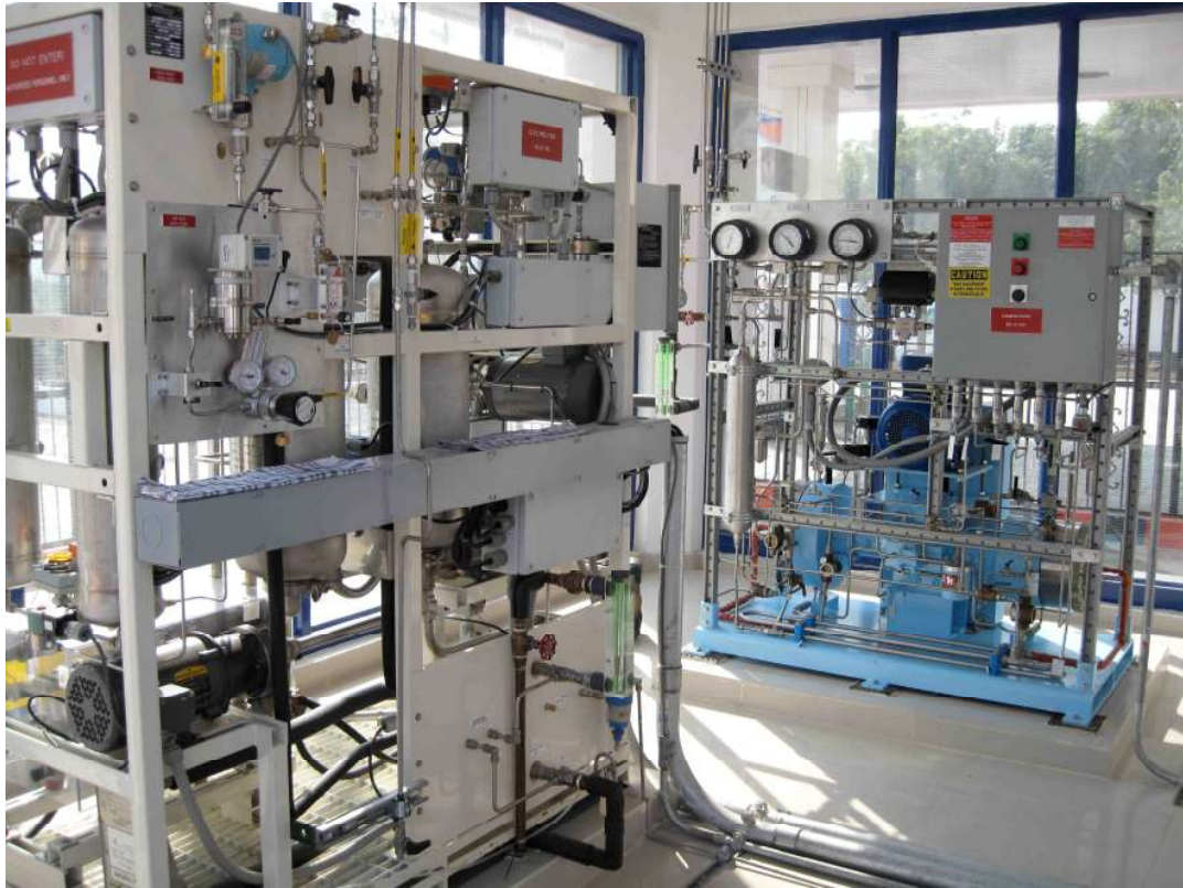
Figure 2 Hydrogen Electrolyser and Compressor built by Eden at Dwarka Station
