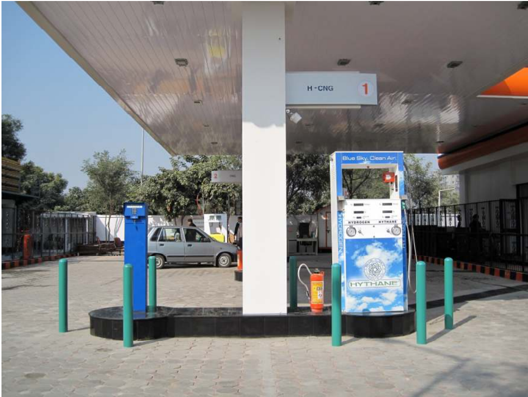
Figure 1 Hythane®/Hydrogen Dispenser at Dwarka Station built by Eden for Indian Oil 2009
