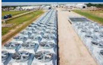
Air Cooled Heat Exchangers (ACHX)
