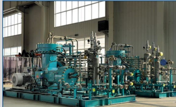
IGAT – part of SIAD GROUP compressor for green hydrogen plant
