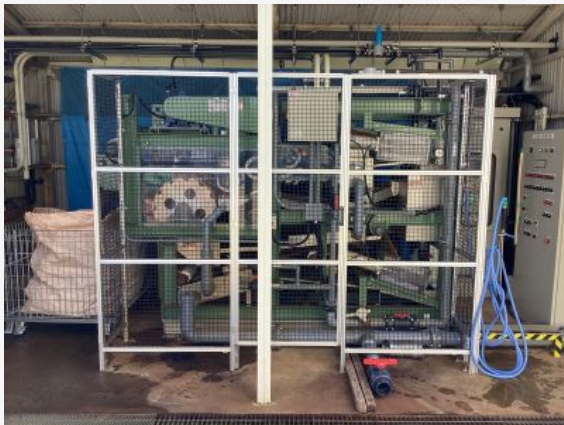
Belt press dewatering machine
