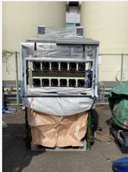
Dewatered sludge dryer
