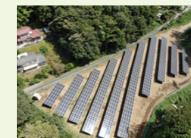
Exclusive SECOM solar power generating facility
