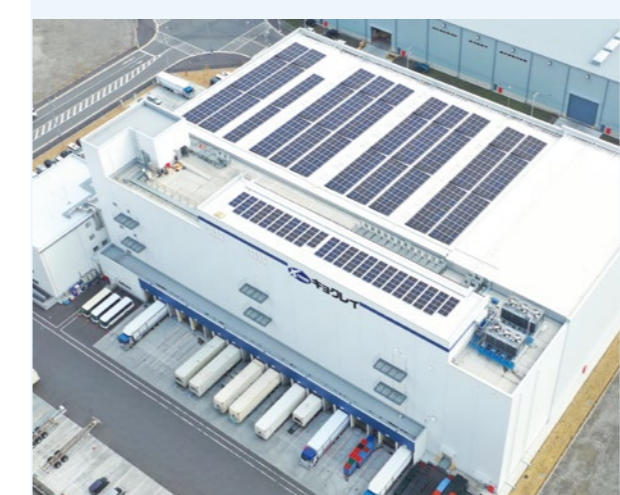
Solar panels installed at the Honmoku Distribution Center of Kyokurei Inc. in February 2022
