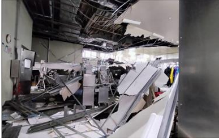
Hokuriku Factory - Ceiling Collapse
