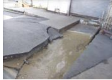
Danchi Factory - Ground Subsidence
