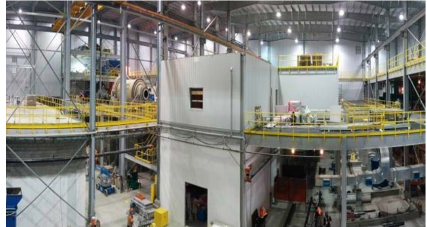
Rubicon Minerals' mill building interior photo, 2014
