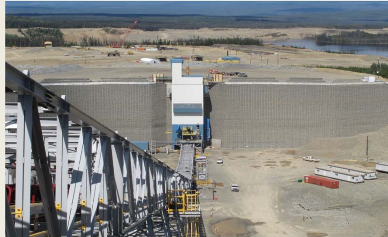
Mt Milligan Primary Crusher
