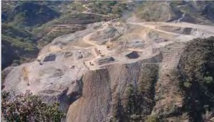
Overview of site preparation work for the Dolores Process Facilities, taken December 2006
