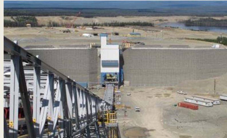
Mt. Milligan Primary Crusher
