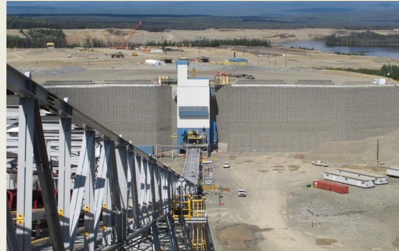
Mt Milligan Primary Crusher
