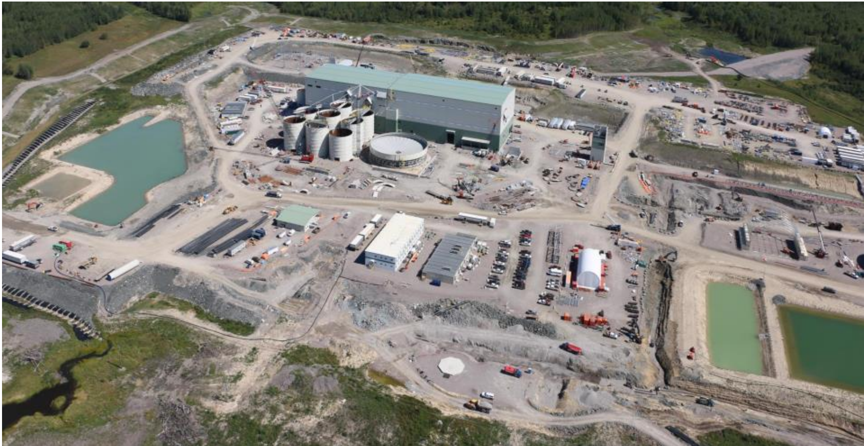
New Gold's Rainy River project is located 65 km northwest of Fort Frances, Ontario. Photo from New Gold.
