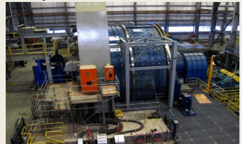
Mt. Milligan Mill Facility
