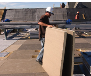
Tapered insulation (above) goes down on a commercial reroof project. With computer-aided design of tapered insulation systems, Beacon is able to design various drainage schemes for its contractors’ projects.
