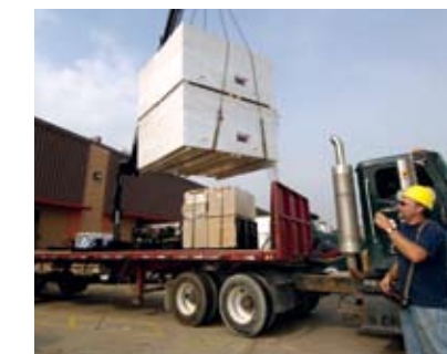
A Beacon flatbed truck crane makes a just-in-time rooftop delivery of materials for a commercial roofing contractor customer near Toronto, Ontario.
