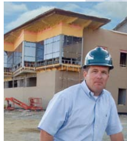
Greg Woods, Waterproofing Specialist in Lancaster, Pennsylvania at a new college sports complex checking the application of the project's vapor/air barrier and the above- and below-grade waterproofing supplied by Beacon.
