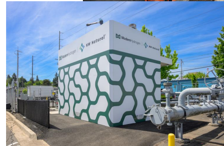
Modern Hydrogen project at NW Natural's Central Service Center
