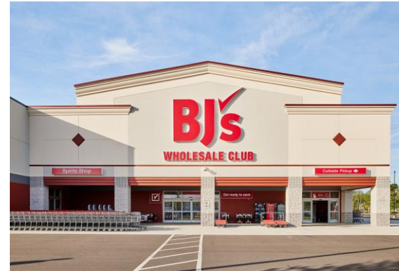
River City Marketplace, Jacksonville, FL 1Q 2024 Completion Demo existing theater box, expand and replace with BJ's Wholesale Club
