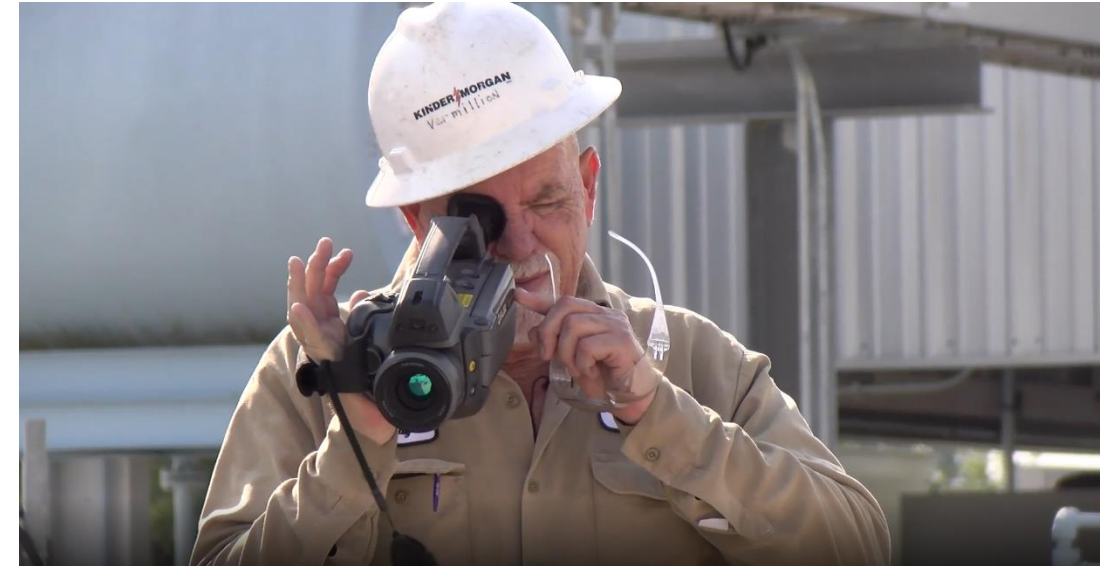
Technician using Optical Gas Imaging to survey for leaks at one of our KM Tejas compressor stations.
