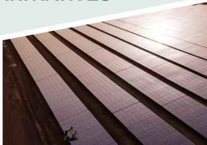
Essakane solar/thermal facility commissioned in 2018 consisting of ~130,000 photovoltaic panels
