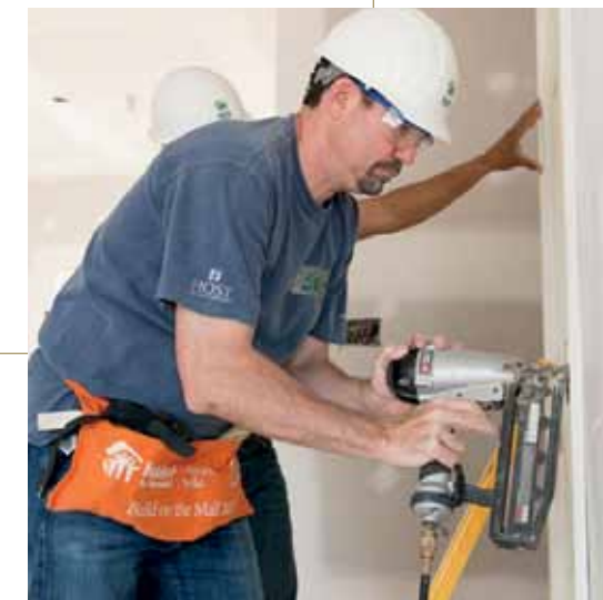
IN 2014, HOST ORGANIZED TWO COMMUNITY BUILD DAYS WITH HABITAT FOR HUMANITY METRO MARYLAND, WHERE EMPLOYEES AND EXECUTIVES WORKED TOGETHER TO COMPLETE CONSTRUCTION ON 19 AFFORDABLE TOWNHOMES IN THE MAPLE HILL TOWNHOME COMMUNITY.
