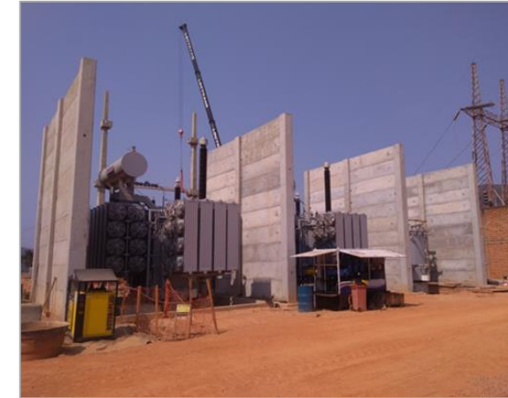
Barreiro Substation (1) Investment of R$ 115 million
