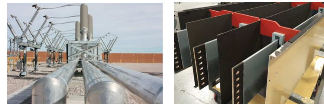
High Voltage Bus
