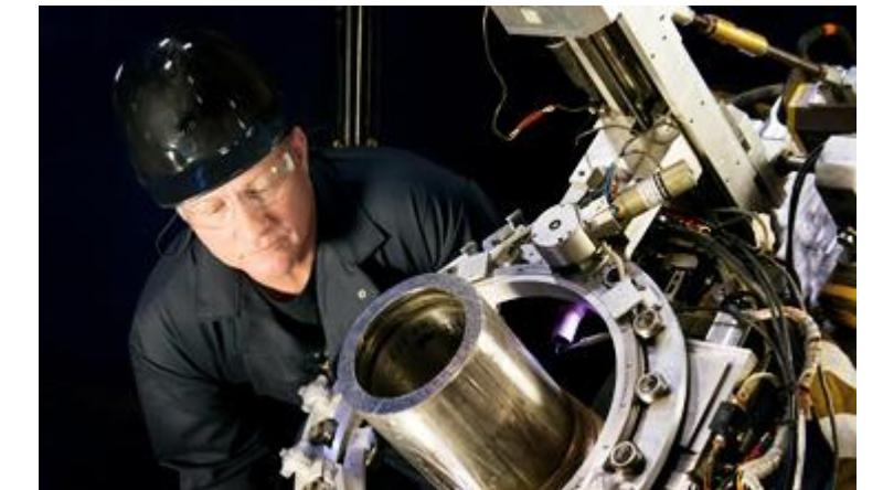
Pipe and Piping Services
