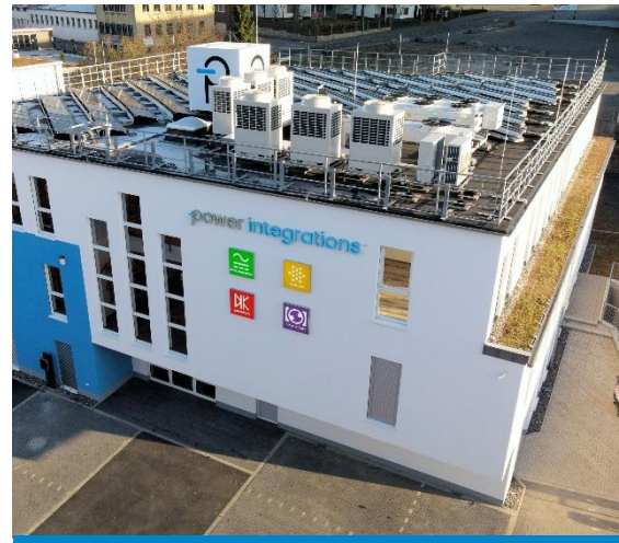
43 kW at New Germany Facility
