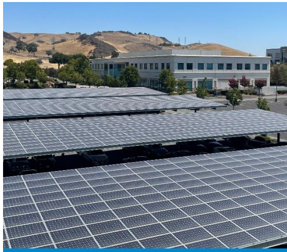
600 kW System at San José HQ
