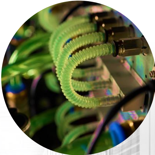
DATA CENTER INFRASTRUCTURE
