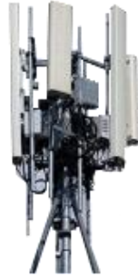
5G Base Station
