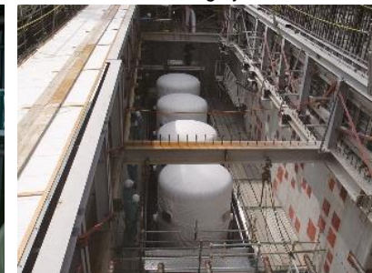
<Filter venting system>
