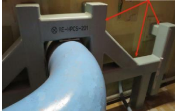
<Support structures (Approx. 10,000 locations)>
