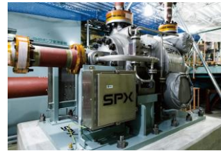
<High-pressure reactor alternate water injection pump>
