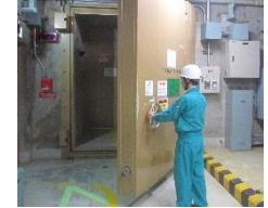
<Watertight doors (59 in total)>
