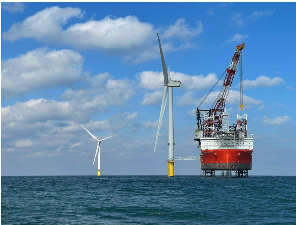
A jack-up vessel performs maintenance works on one of the five Blyth 1 offshore wind turbines located in Blyth, Northumberland.
