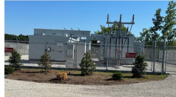
New Foristell substation energized in May 2024 to support reliability for nearly 3,000 customers
